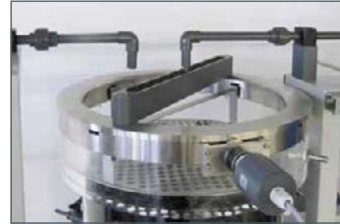
Rotary distributor on the head of the trickling filter with variable speed adjustment
