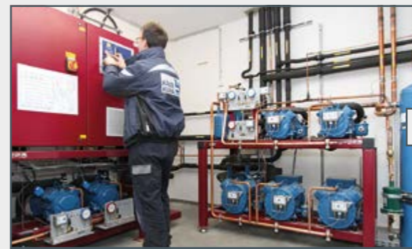
Industrial refrigerating plant
